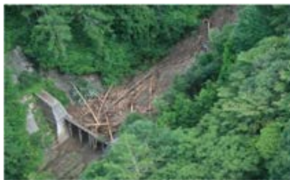
4号格子型えん堤被災状況 h=8m, L=45m, h21
